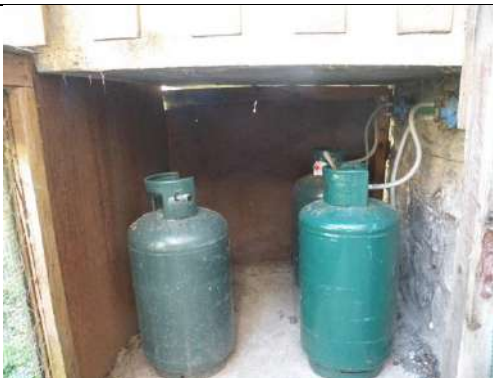
18. Bombole gas in esterno
